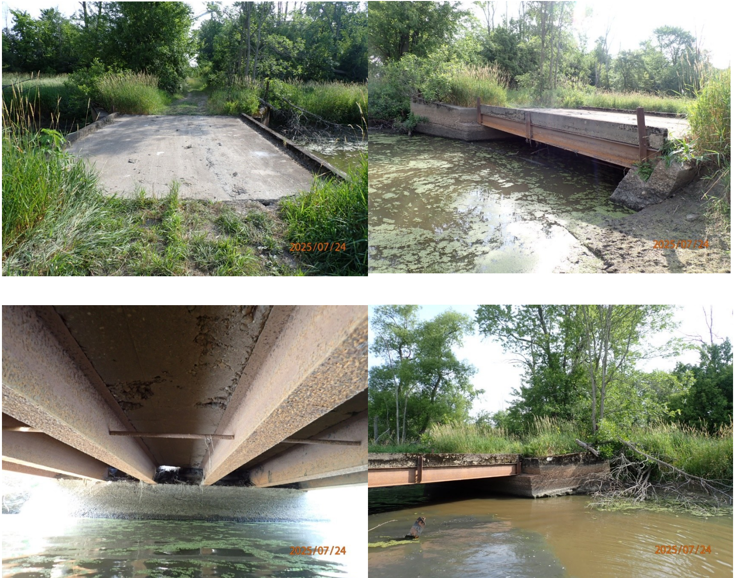
Figure 95 Photos of a culvert in 'very poor' condition: Baldwin Road Bridge
